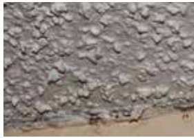
Asbestos coated ceiling.
