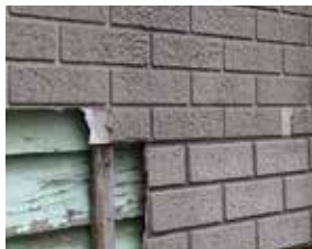
Asbestos veneer cladding covering weatherboards.
